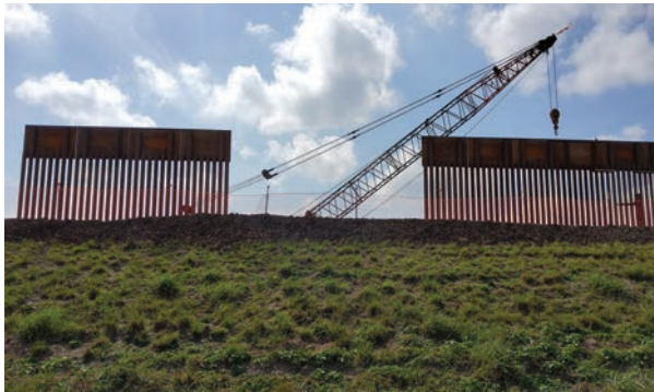
AFP's Mark Anderson snapped this photo of a portion of border wall being constructed near Donna, Texas, in an area formerly known as "Drug Alley."
